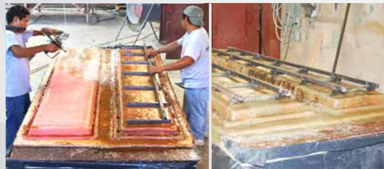
4 After all layers are cured, a mother mold made of fiberglass and resin is applied using a chop gun. Steel tube stock is added to strengthen and support the shell.
