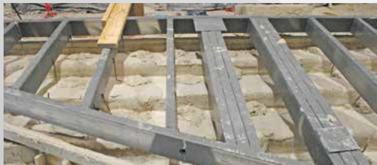
6 Pre-welded steel flex anchors attach the frame to the GFRC skin, using GFRC bonding pads.
