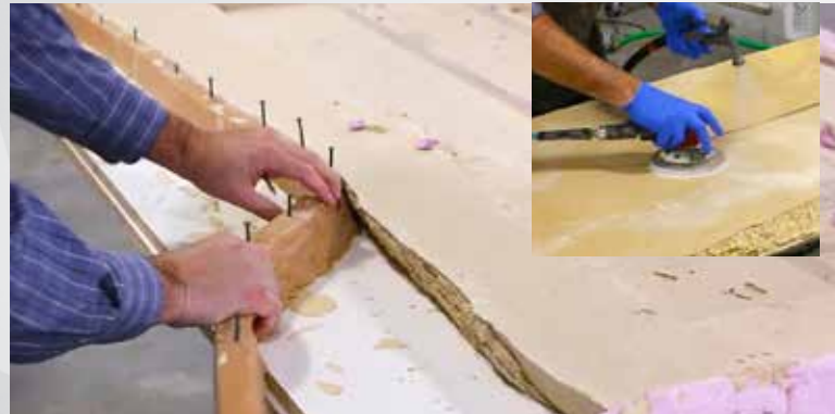
4 After curing for 16 hours, the molds are removed, revealing the textured edges. The table top is wet polished using diamond pads.
