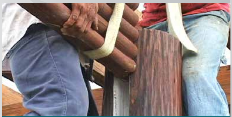
12 Once cured, artisans align lightweight GFRG bamboo panels with pre-fabricated channels in the columns which makes placement easy.
