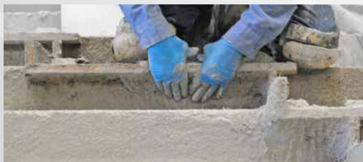
4 Additional backup mix is applied by hand to reinforce corners, edges, and reveals.
