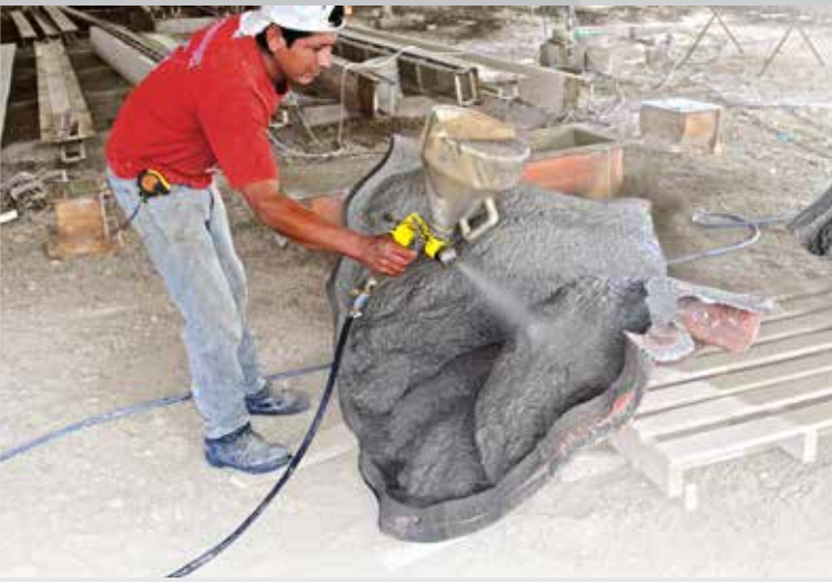
5 GFRC is sprayed into the mold halves. Mold halves are then put together.
