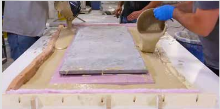
3 ECC Blended Mix™ is poured into the mold and spread by hand, then troweled level.
